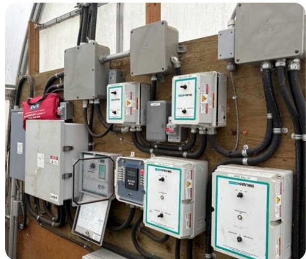
Figure 12. Electrical panel and automation system at Twin Sisters Native Plant Nursery.
