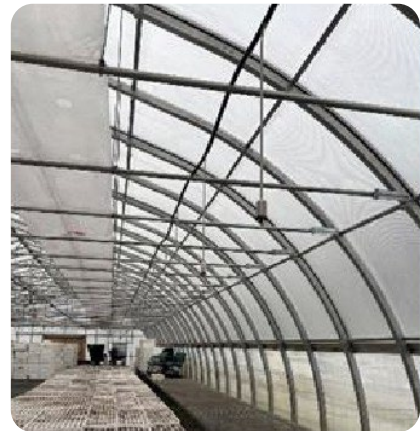
Figure 1. Overhead irrigation system at Twin Sisters Nursery.
