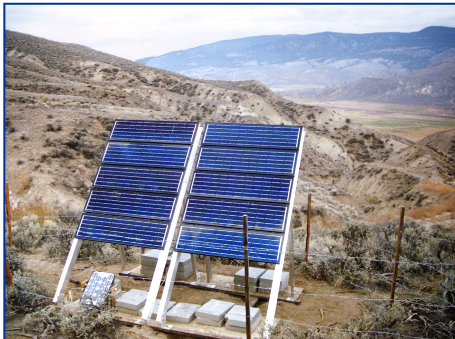
Figure 1 A Ten Panel Photovoltaic Array
