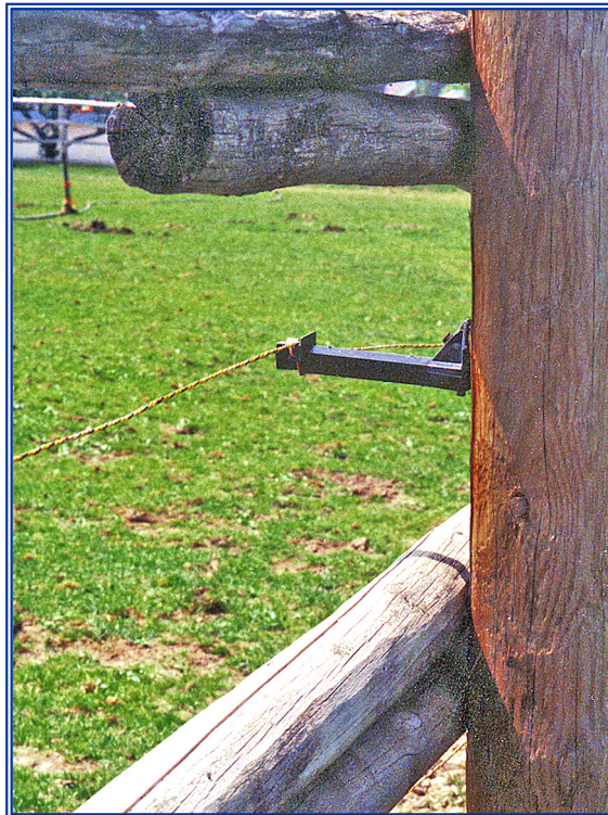
Figure 3 Typical Offset Line Post Insulator
