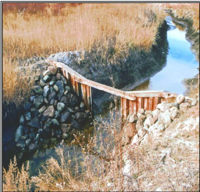
SHEET METAL WATER CONTROL STRUCTURE
