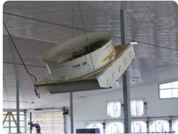
Figure 4. “Cyclone” style fan used to blow air into the free stall area.
