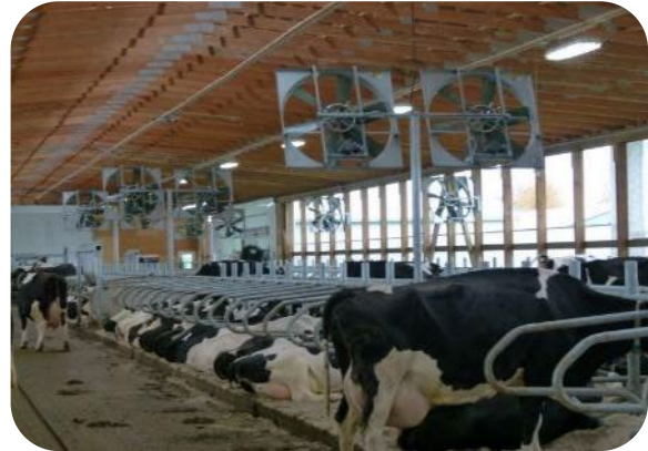
Figure 1. Place fans over free stalls to direct the air into the cow resting area.
