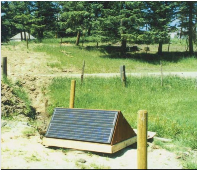
Figure 3 100 Watt PV Water Pumping System
