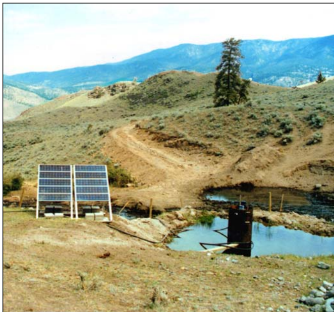
Figure 1 500 Watt PV Water Pumping System
