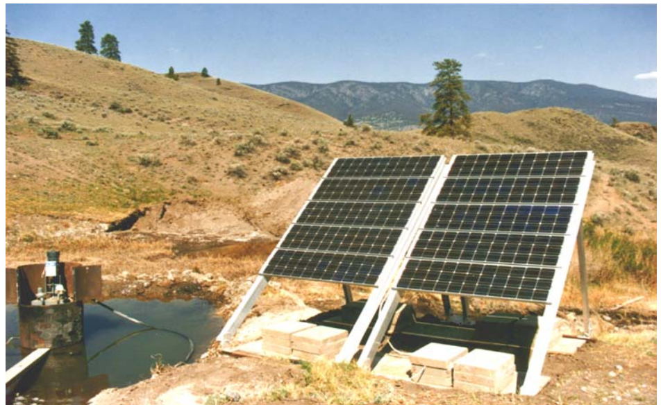
Solar-Powered Pump Using Photovoltaic Panels
