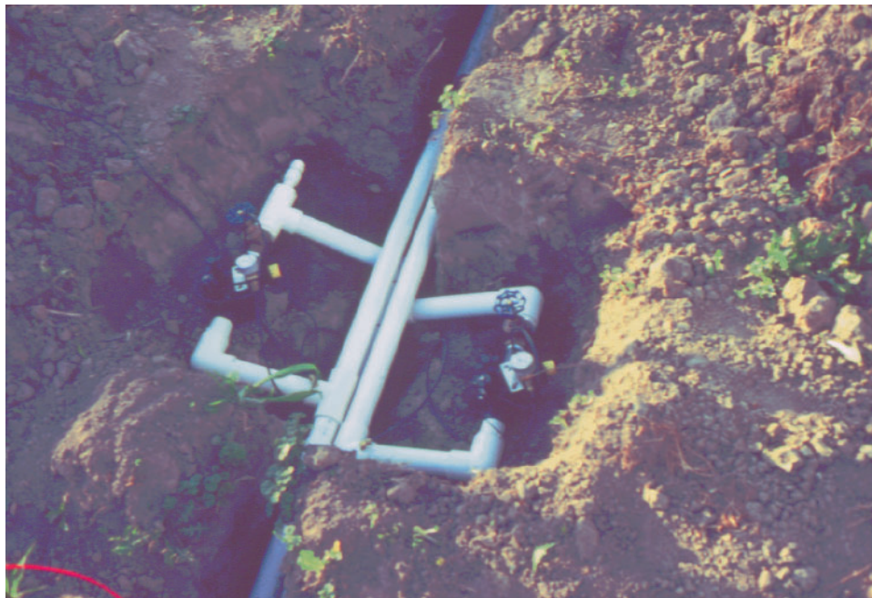
Control Valve Installation on Sub-main
