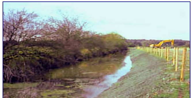
Figure 4 Fence on a Recently Hydro-seeded Channel
