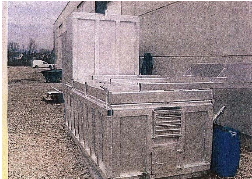
Figure 4.1: Picture of Inciner8 Model 2600(HF) Incinerator
