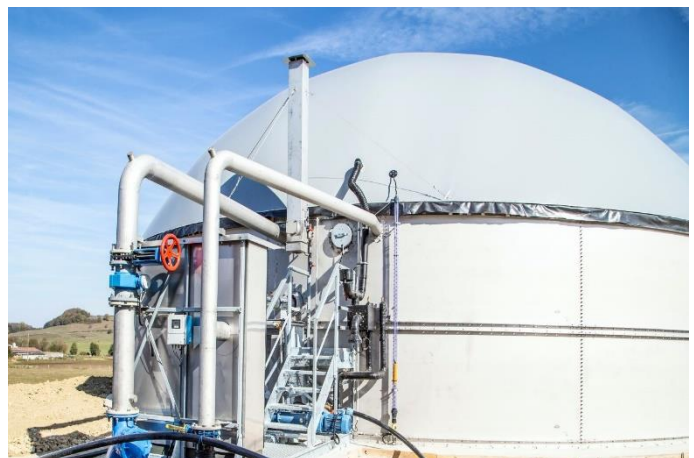
Example of a PlanET Biogas modular biogas plant. Source www.planet-biogas.ca
