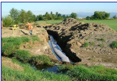
Figure 5 Diversion Channel with Pipe to Reduce Erosion
