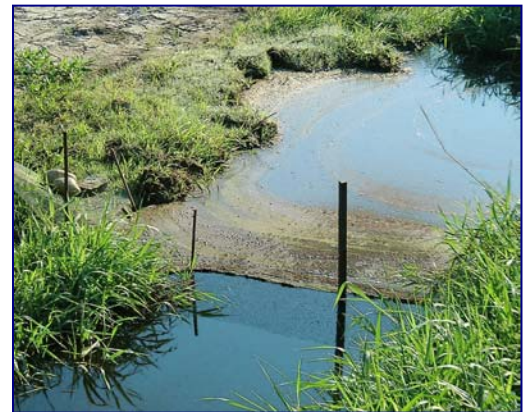
Figure 10 Temporary Silt Fence
