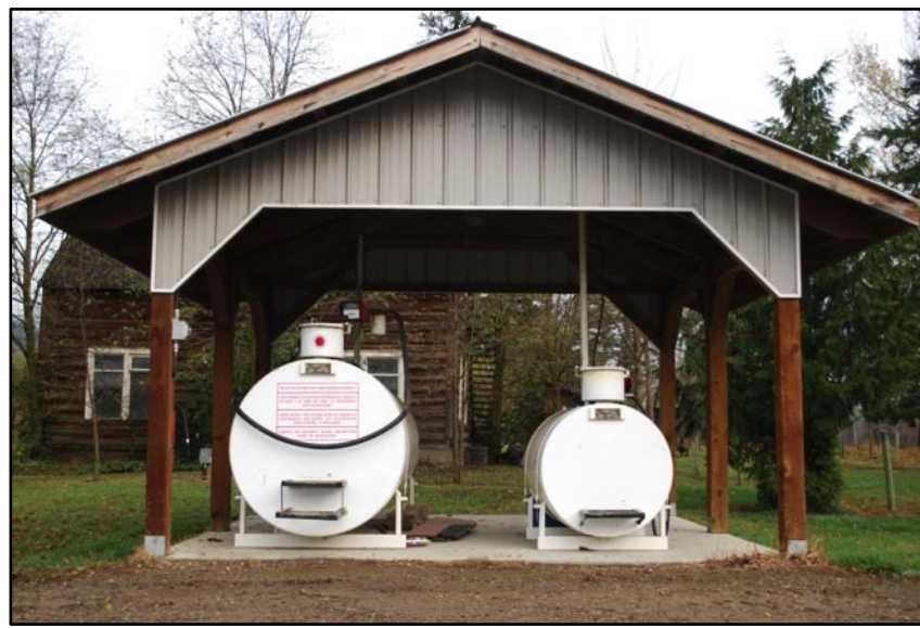
Figure 14: Fuel Storage BMP including double-walled tank and roof
