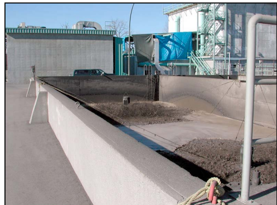
Photograph 8: Aerobic digester at the Langley WWTP
