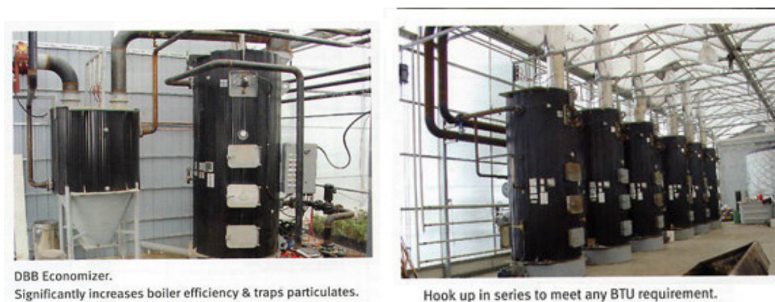
Figure 10: Decker Manufacturing Greenhouse Boilers
