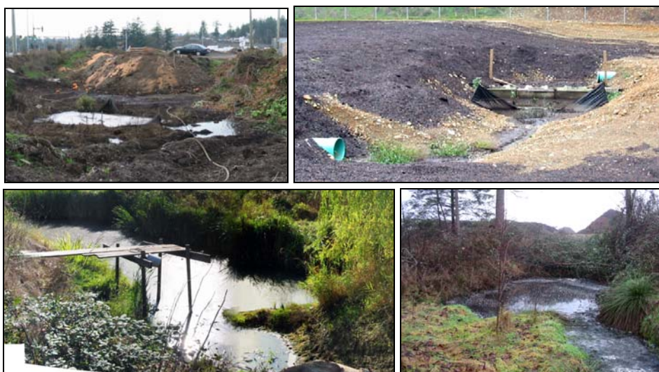
Figure 5 Leachate collection ponds at various sites. EPO's inspection assessments were that ponds are generally poorly constructed and/or maintained as there is no documentation that the underlying soil is impermeable and/or they appear to overflow in wet weather.
