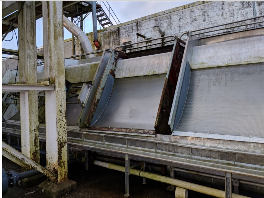
Photo 1 – Series of 5 wedge wire screens for effluent with 25 mesh fine screening.
