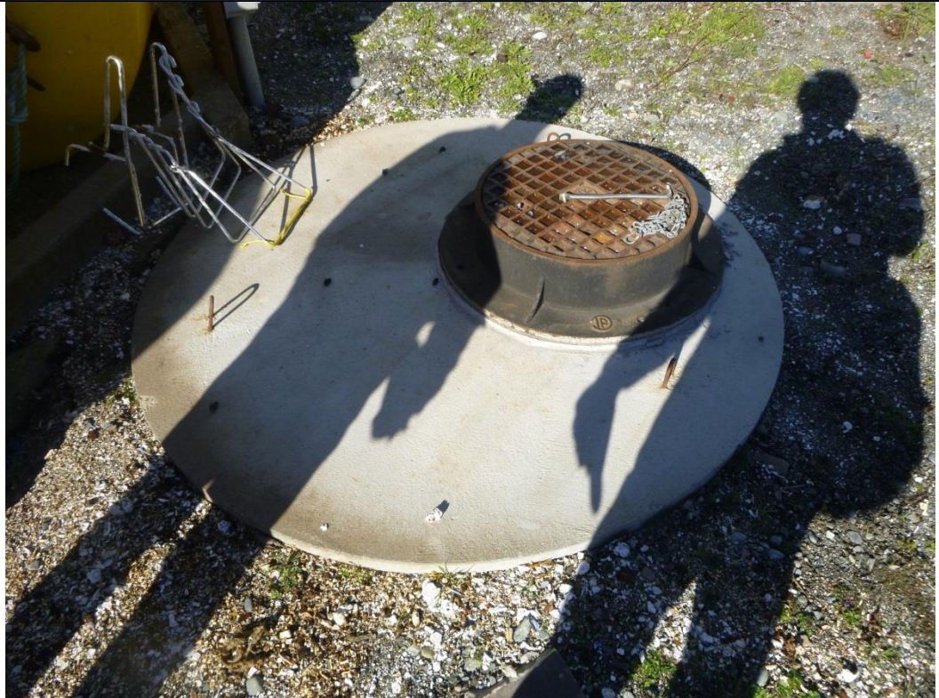
Photo 2 Underground wastewater collections sump that pumps up to the above ground tank.
