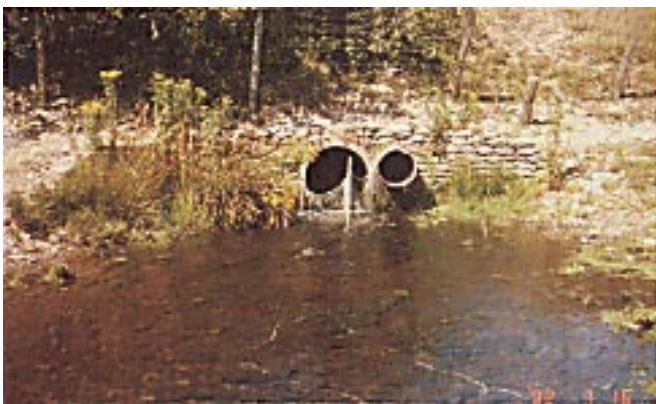
IMPROPER CULVERT INSTALLATION BLOCKS MOVEMENT OF FISH.
