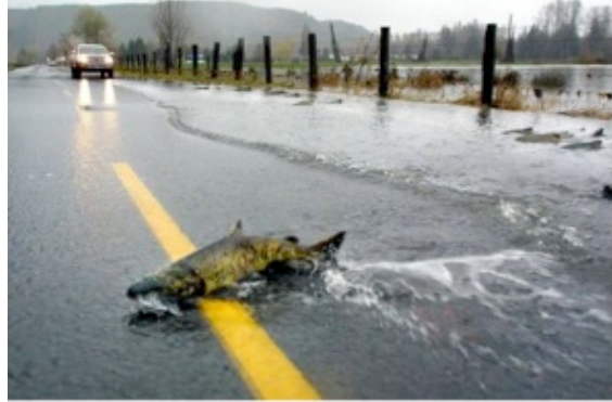
Why is the fish crossing the road? Because the culvert is impassible
