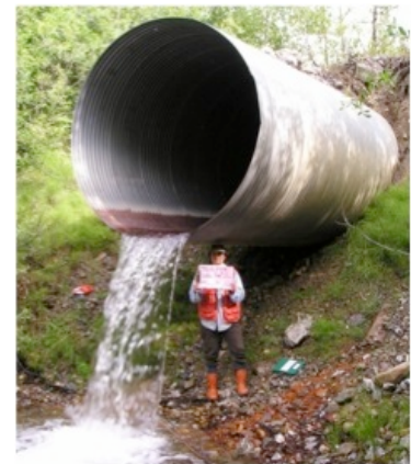
A culvert with a vertical drop at its outlet making it impassable to fish
