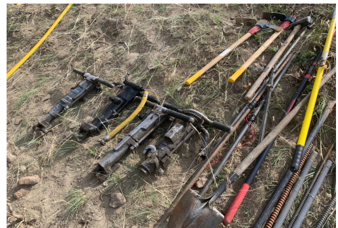
Pneumatic drills, pictured left, are used by rock scalars to assist with rock removal at the slide site.
