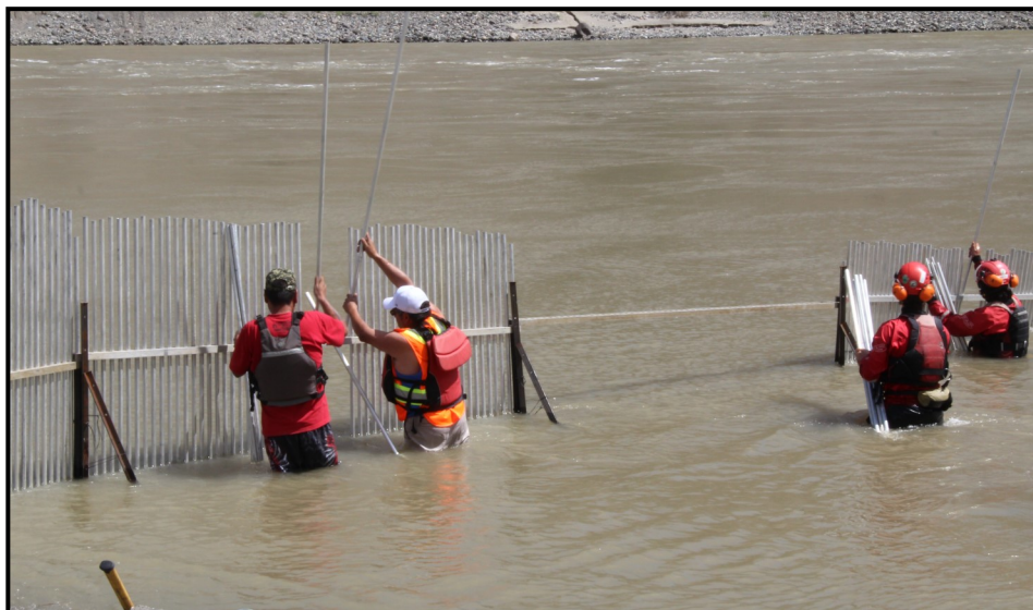
PICTURED: Northern Secwepemc Tribal Council fisheries staff, along with a Swift Water Rescue crew worked to install the picket weir for the off-channel holding pond in 2019.
