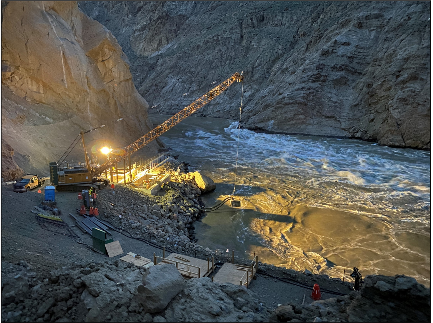
PICTURED: Pumps for the concrete fish ladder being placed in the river by crane.
