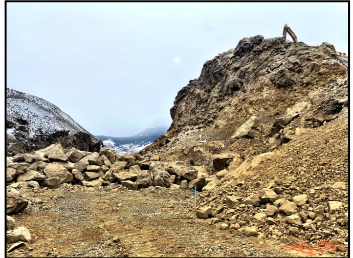
TOP: Materials for the permanent fishway foundation and the new "nature-like" fishway are being processed on the East Razorback.
