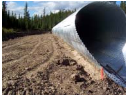
Figure 10. Assembled culvert showing clay material placed next to the culvert and above the lowest bolt holes (photo courtesy of Alberta-Pacific).
