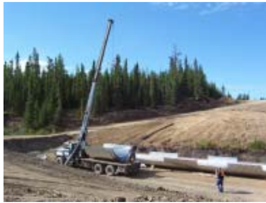
Figure 9. Truck with extended crane to lift pre-assembled sections into place during construction. Note the sections on the back of the truck (photo courtesy of Alberta-Pacific).
