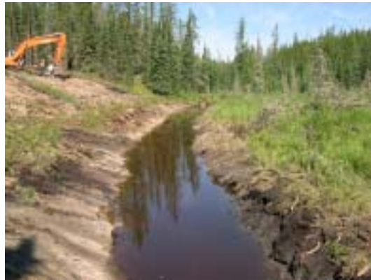
Figure 3. Looking downstream along the open diversion trench (before the decision was made to use round culverts).
