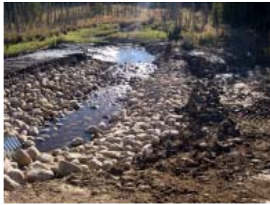
Figure 14. Inlet of culvert showing length of reconstructed stream channel, size and amount of rock, and stream-riffle section near the end of the armoured streambanks.
