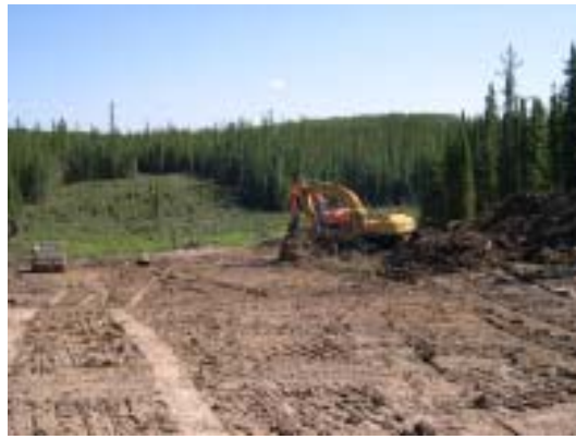
Figure 1. View of the wetland depression and right-of-way clearing on far side of crossing.
