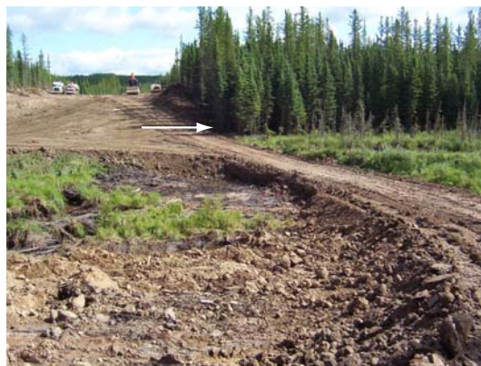
Figure 5. Tote road which allowed equipment to pass the culvert installation site. Arrow shows the abrupt and distinct boundary between the wetland area and forested area (photo courtesy of Alberta-Pacific).
