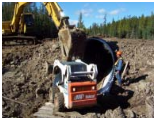
Figure 13. Excavator placing infill material into the bucket of the front-end loader during the infilling of the culvert (photo courtesy of Alberta-Pacific).
