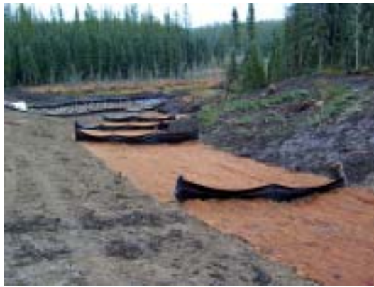
Figure 18. Fibrous matting and geotextile fences placed across ditchline (photo courtesy of Alberta-Pacific).
