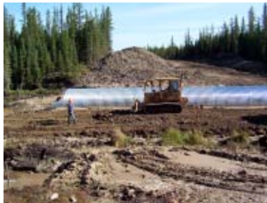
Figure 12. Crawler tractor spreading backfill material. Note the large pile of excavated material on the far side of the culvert (photo courtesy of Alberta-Pacific).
