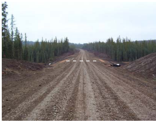
Figure 20. View of road surface across the installed culvert (photo courtesy of Alberta-Pacific).
