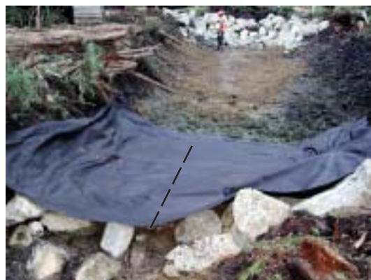
Figure 3. Prepared excavation showing the use of riprap at either end, a layer of bedding material through the length, and geotextile before being cut. Dashed line shows approximate cut line.
