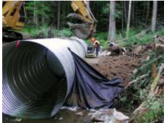
Figure 8. Forest worker attaching plate compactor to excavator's bucket hook in preparation for lifting it to the other side of the culvert. Notice the geotextile tied over the top of the culvert.
