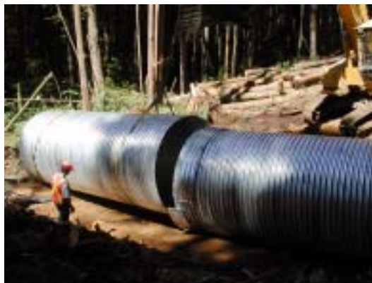
Figure 6. Second section of the culvert being dragged towards the first section using a single lifting strap. Notice the section of the coupler below the culvert.
