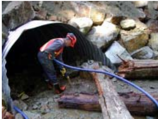
Figure 11. “Washing” the staging area near the inlet of the culvert. Note the large woody debris.
