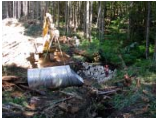
Figure 4. Lifting straps were used to carry the inlet section of the culvert.
