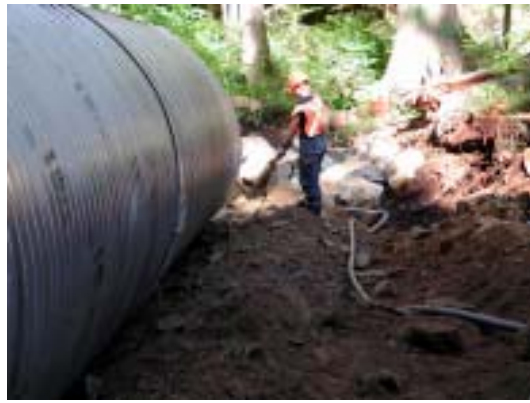
Figure 7. Forest worker using pumped water to force backfill material below the haunch of the culvert.
