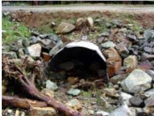
Figure 12c. Inlet of embedded culvert showing height of fill, riprap armouring, and use of woody debris.
