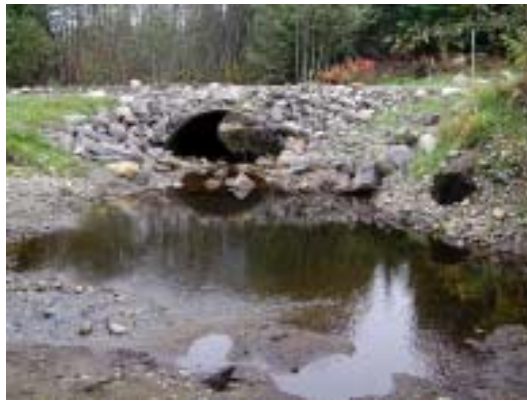
Figure 2b. Culvert inlet showing pool area and shallow fill height above culvert.
