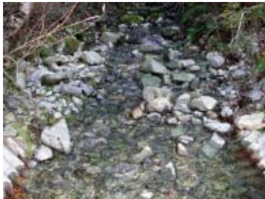
Figure 1c. Culvert inlet showing match to natural stream width and gradient.
