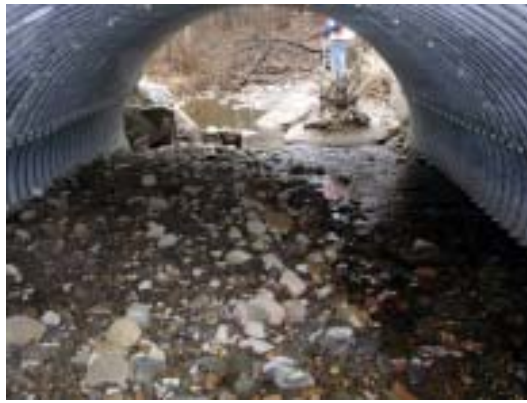
Figure 5b. Looking downstream through the embedded culvert, showing the stream flowing along one side of the culvert at this location.
