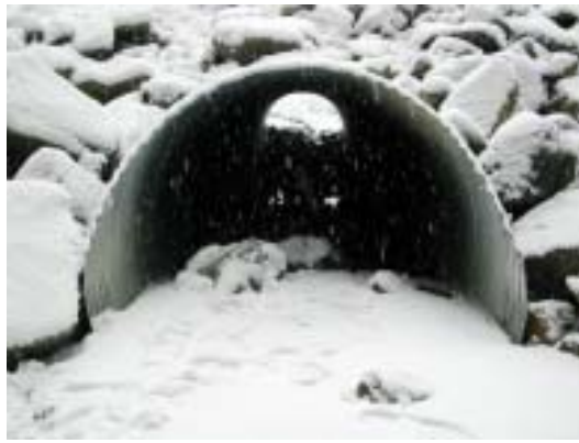
Figure 10b. Looking upstream showing the size of larger material within the culvert and riprap armouring of the fill slope.
