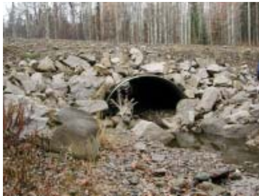
Figure 5c. Outlet of embedded culvert showing height of fill, riprap armouring, and a small root wad deposited during high flows.
