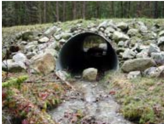
Figure 11c. Inlet of embedded culvert showing width of natural stream and undisturbed stream banks.
