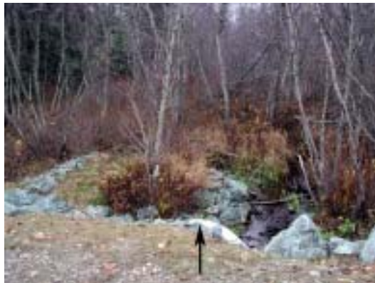
Figure 3c. Looking downstream from culvert outlet showing deciduous forest, and rock spur on left hand side of image (arrow indicates obvert/top of outlet).
