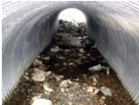
Figure 10a. Looking towards the culvert inlet, showing simulated streambed one year after installation.
