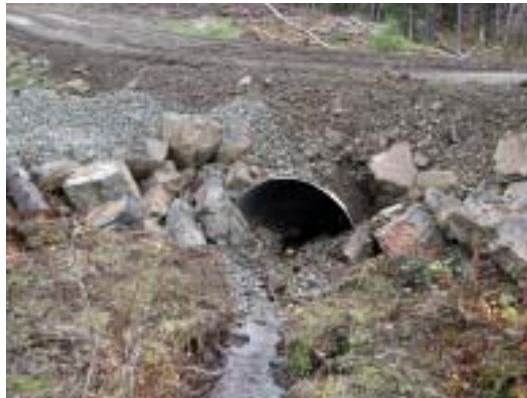
Figure 7c. Inlet of embedded culvert showing riprap armoring, use of drain rock along the ditch and fill slope, and minimal disturbance to natural streambank.
