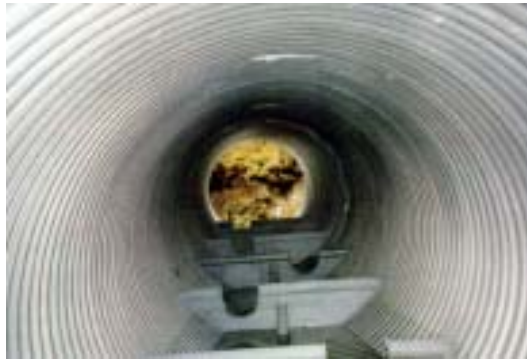
Figure 12b. Embedded culvert before placing material within it, showing height of baffles (photo courtesy Weyerhaeuser, Stillwater Timberlands).
