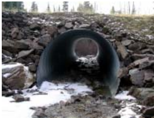
Figure 9c. Inlet of culvert showing riprap armouring and height of fill over the culvert.
