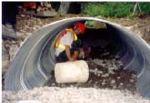
Figure 7b. Worker delivering material within the culvert during installation (photo courtesy of Canadian Forest Products Ltd., Fort St. James).
