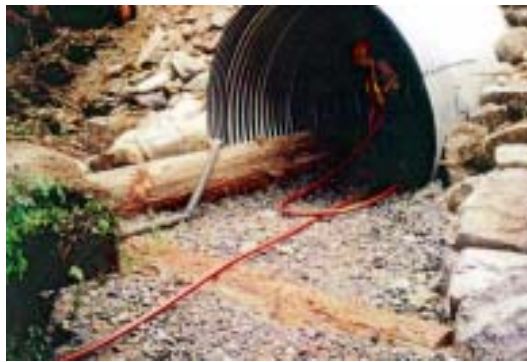
Figure 11b. Outlet of embedded culvert, showing woody debris placed within the culvert and worker conducting final wash of simulated streambed (photo courtesy Weyerhaeuser, Stillwater Timberlands).
