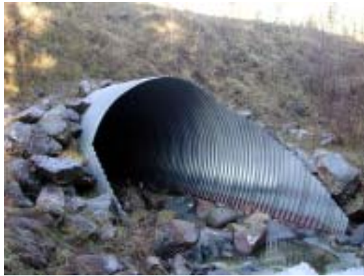
Figure 8c. Inlet of culvert showing step-bevel and high water markings along culvert wall.
