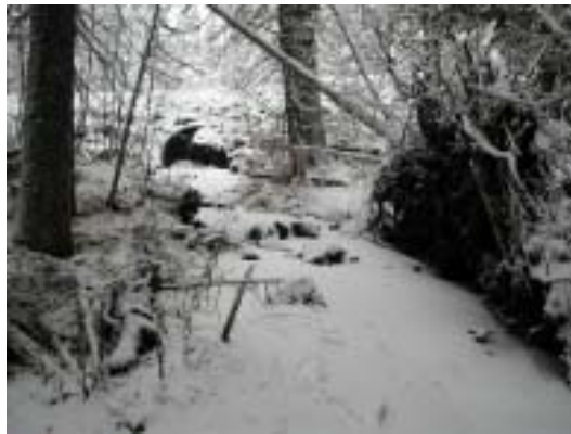
Figure 10c. Looking upstream towards embedded culvert showing stream channel, height of fill above culvert, and road grade.
