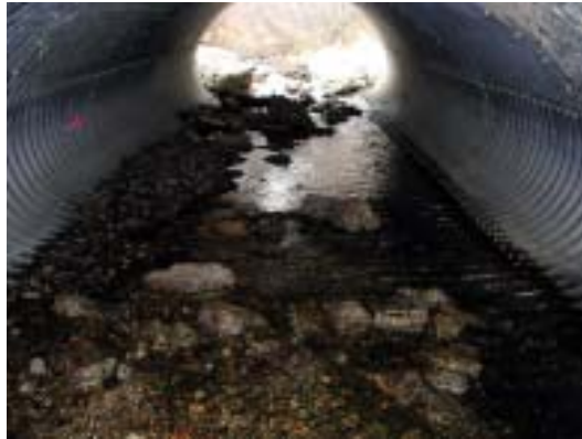
Figure 6c. Embedded culvert showing boulders intermingled with natural deposits of sand and gravel.
