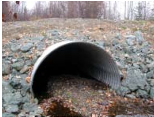
Figure 4b. Inlet of embedded culvert showing leaf litter and gravel material placed within the culvert.
