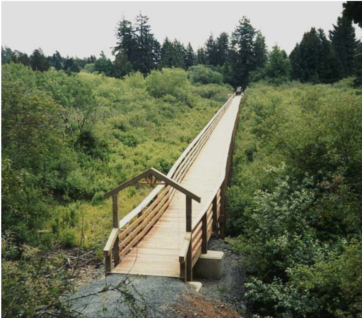
Plate 5: Polygon C0724 - Wetland Disturbed by boardwalk in greenspace. Note the trimming that occurred when the boardwalk was built. The boardwalk also creates a patch of shade which will inhibit the growth of some plant species and may act as a barrier to the passage of some animals, especially when the boardwalk is heavily used by people. However, utilization of a boardwalk does minimize uncontrolled access which could be even more damaging.
