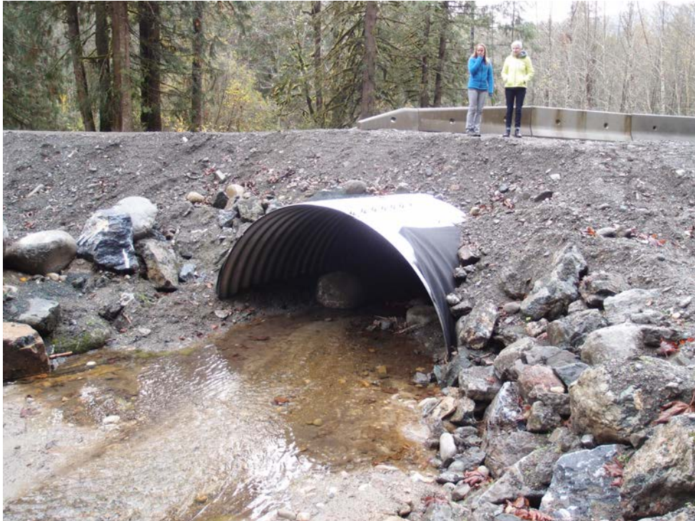
photo: Newly installed open bottom arch culvert that provides for safe fish passage
