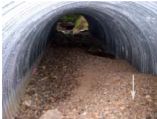
Figure 1c. Mound of gravel (white arrow) along one side of the culvert near the inlet.
