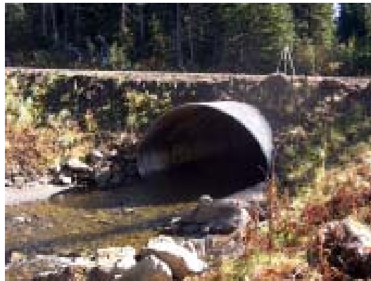
Figure 4c. Outlet of embedded culvert showing riprap armouring on the right, riffle area near the outlet, and shallow road fill above the culvert.
