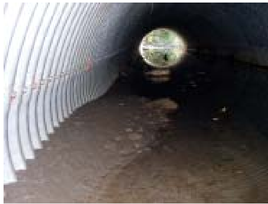
Figure 2c. Embedded culvert showing finer, sandy material deposited along one side of the culvert's inlet. The opposite side is mostly bare.
