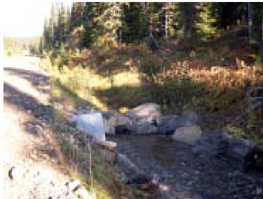
Figure 3c. Inlet of embedded culvert showing stream turning sharply into the culvert.
