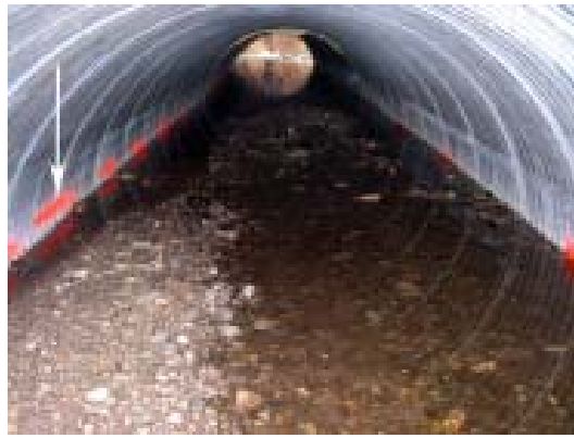
Figure 7a. Looking towards outlet of embedded culvert, showing predominantly gravel substrate. Spray paint lines, as indicated by the arrow, along the culvert's wall indicate target infill depth plus 5 cm.
