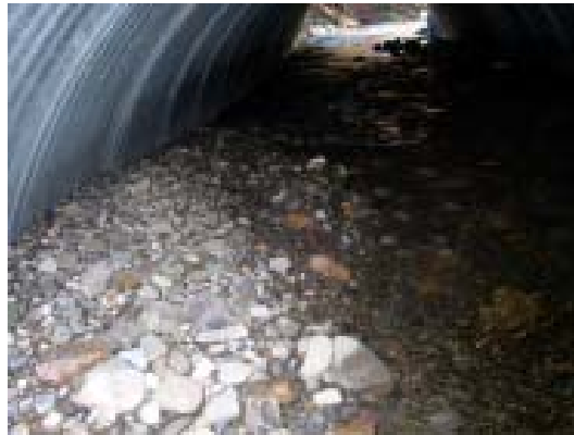
Figure 3b. Inlet of embedded culvert showing uneven depth of aggregate partly due to the stream turning sharply into the culvert.
