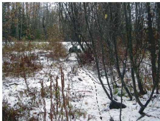
Figure 6c. Looking towards the outlet of the embedded culvert, showing flat terrain and shallow stream banks (dashed line indicates the approximate centre of the stream channel).
