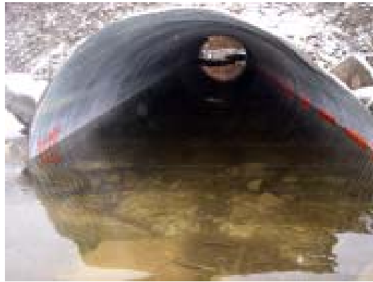
Figure 7b. Outlet of embedded culvert showing water depth during field visit and subsurface material.
