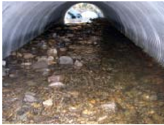
Figure 3a. Looking towards inlet of embedded culvert, showing stream flow and cobble sized material.
