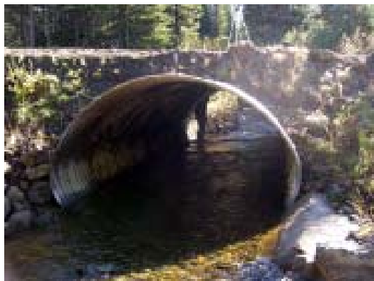
Figure 4a. Looking upstream showing the embedded culvert, stream flow, and one partially exposed baffle.
