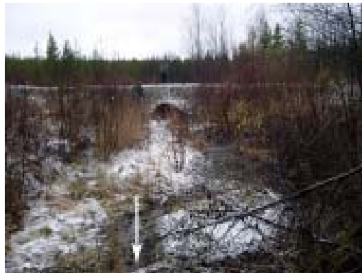
Figure 7c. Looking towards the outlet of the embedded culvert showing flat terrain and shallow stream banks. Arrow indicates centre of braided stream channel through the powerline clearing.
