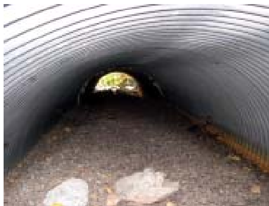
Figure 5a. Looking towards outlet of embedded culvert showing surface cobbles and gravel.
