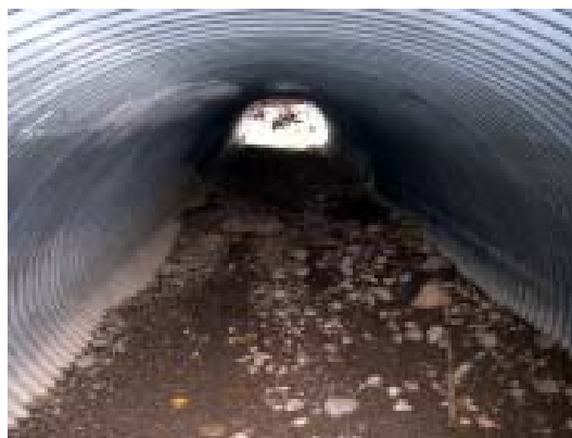
Figure 6a. Looking towards inlet of embedded culvert showing sandy bottom with surface cobbles and gravels.
