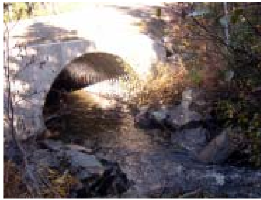
Figure 4b. Inlet of embedded culvert showing concrete headwall and riprap armouring along the stream bank.
