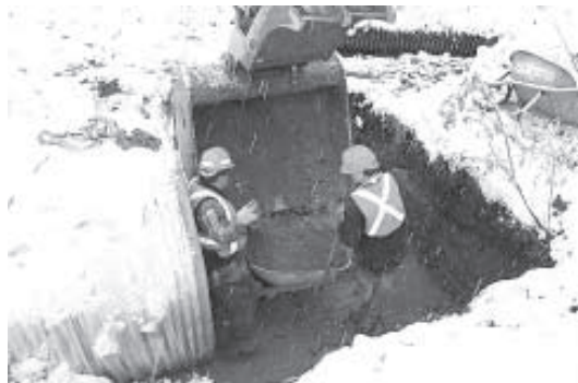
Figure 9. Embedding crew filling wheelbarrows at inlet end of CSP. (Photo courtesy of Brian Chow, BCMOF.)
