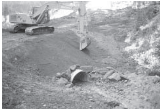
Figure 13. Excavator grading the final road fill at inlet of embedded CSP. Notice the final placement of the riprap armouring.
