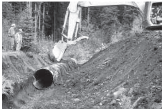
Figure 4. Excavator removing coupler between two sections of the existing 900-mm CSP. Notice one section has been removed already.
