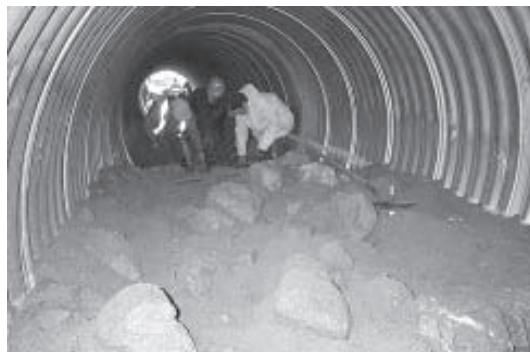
Figure 10. Forest workers mixing material within the CSP. Note fill-height line spray painted inside CSP. (Photo courtesy of Brian Chow, BCMOF.)
