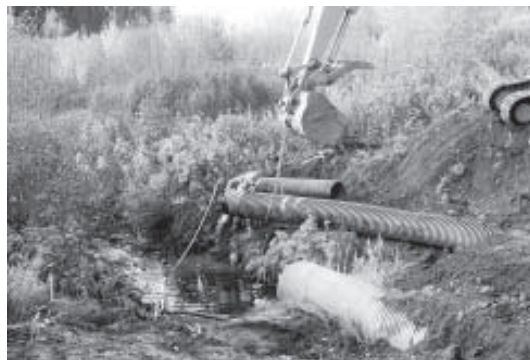
Figure 3. Forest worker preparing diversion pipe (being lifted by excavator) in preparation for adding an additional section.
