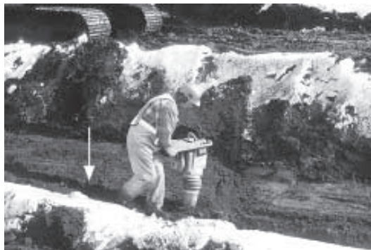
Figure 8. Jumping-jack compactor. Notice the swath to the left of the forest worker (arrow) compacted during one pass.
