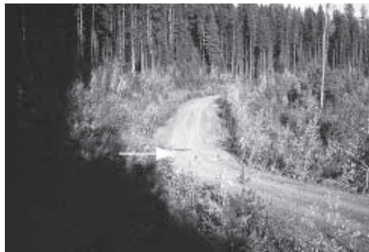
Figure 1. View of installation site before construction. Arrow indicates where existing CSP passes through the road.
