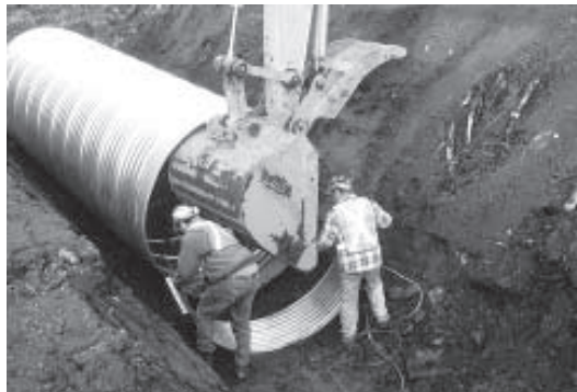
Figure 6. Excavator lifting one end of the CSP while forest workers place the bottom side of a coupler under it.
