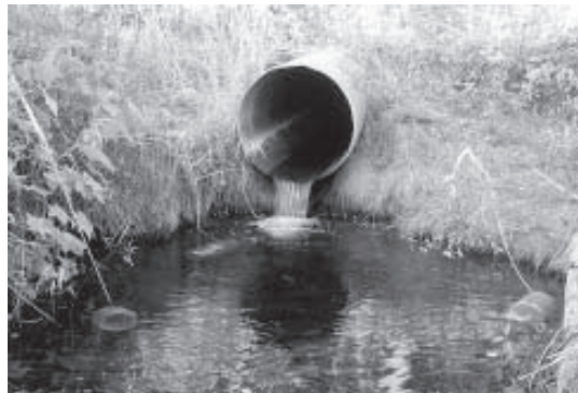
Figure 2. Outlet of the existing CSP showing the fish barrier and fish traps placed in the plunge-pool.
