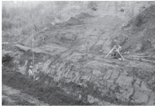
Figure 5. Surveyor checking depth of excavation along the length of the prepared trench.
