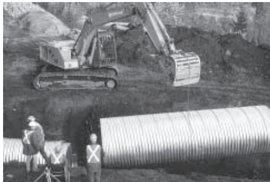
Figure 7. Excavator lowering second section of CSP into place. Notice bottom section of coupler in place below the stationary section of CSP.
