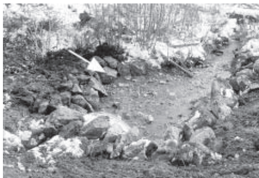
Figure 11. Final installation at downstream side of CSP showing riprap armouring and location of splash-pad (arrow).
