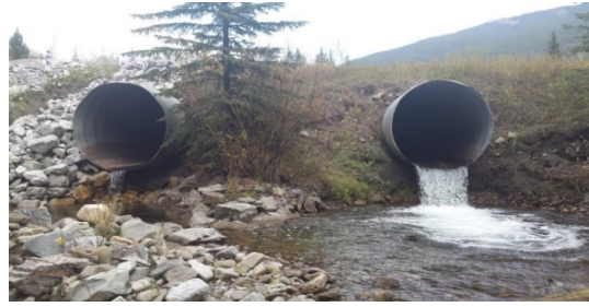
Figure 11 Unmaintained culvert on Chauncey Creek in the Elk Valley, demonstrating a closed-bottomed culvert that prohibits fish movement upstream (photo: Taye Ayele).
