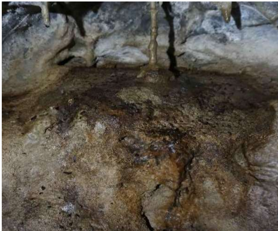
Figure 49. Staining from roosting bats. (Photos: Martin Davis)
