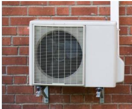
Heat Pumps and PTHPs
