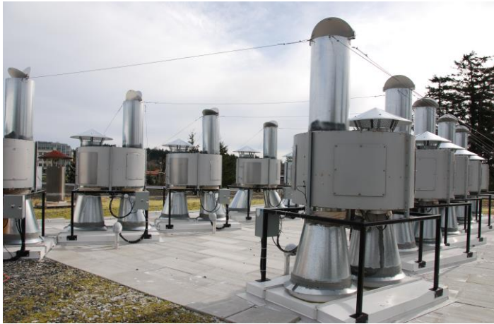
Victoria Regional Laundry – Dryer Heat Recovery Project $210,000 – Custom Retrofit Program Incentive
