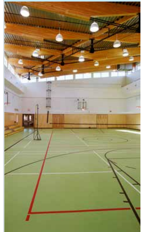
Image 3: The roof of the gym at the Doig River Community Centre features glulam beams with steel tension rods to create an aesthetically striking and efficient design (Image courtesy of Equilibrium).
