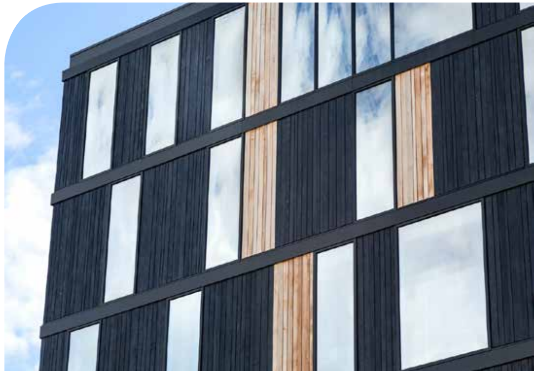
Image 5: The Wood Innovation Design Centre at the University of Northern BC in downtown Prince George used the Shou Sugi Ban technique of creating a durable charred wood finish (Image courtesy of Ed White).
