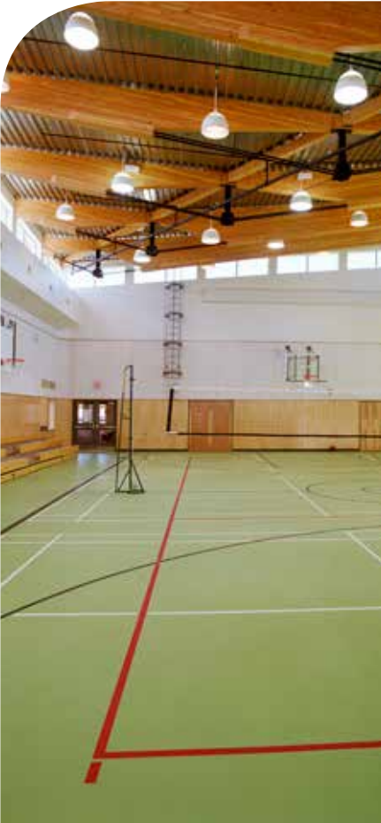
The roof of the gym at the Doig River Community Centre features glulam beams with steel tension rods to create an aesthetically striking and efficient design (Image courtesy of Derek Lepper).
