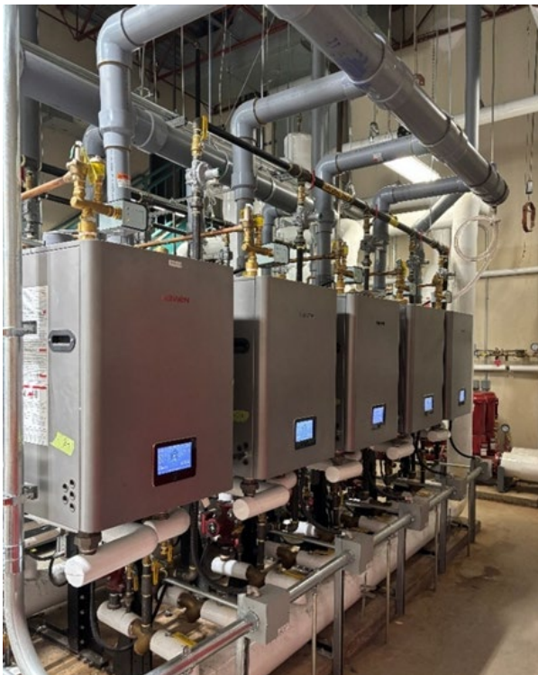
SARDIS SECONDARY BOILER PLANT
