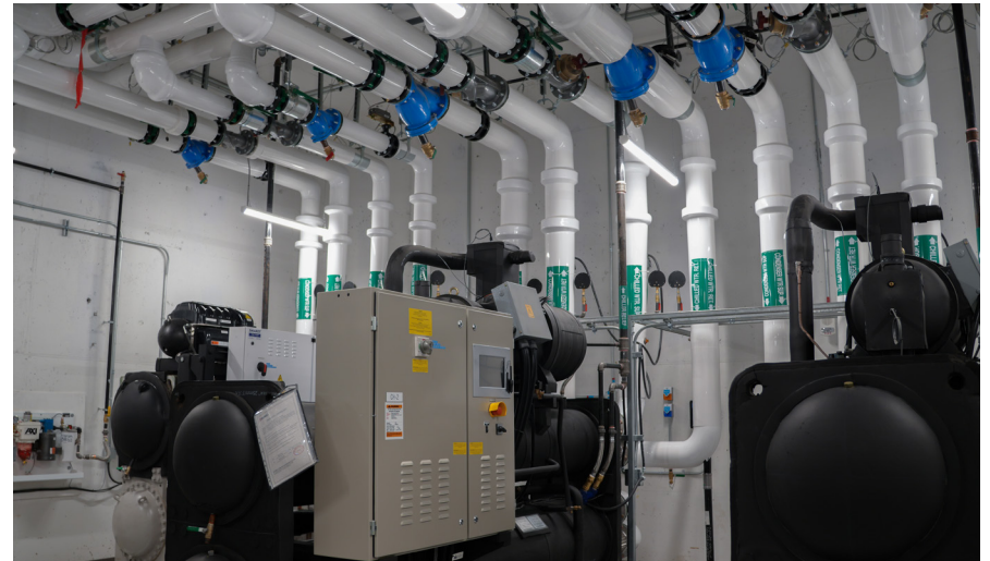
Efficient heat recovery chillers at Nats'oojeh Hospital and Health Centre, Fort St. James
