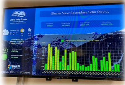
Figure 1 – Glacier View Secondary PV Array Control Panel
