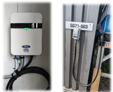
Figures 9&10 – BEV Charging Station
