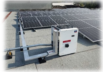
Figure 4 – Glacier View Secondary Rooftop PV Array
