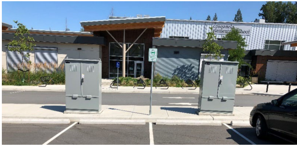
EV Chargers at Casqanelo Elementary
