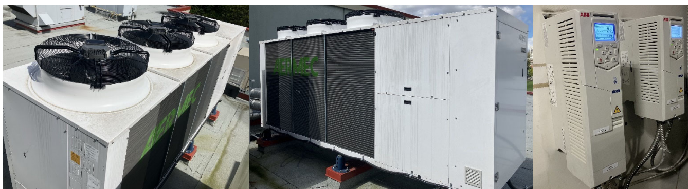
Glenbrook Heat Pump
