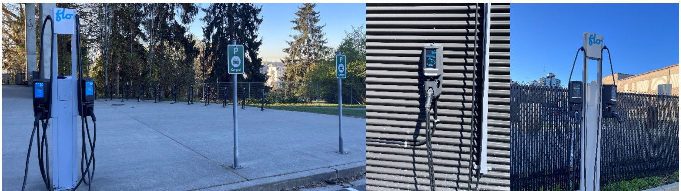
EV Charging Stations & carpool parking in School District 40
