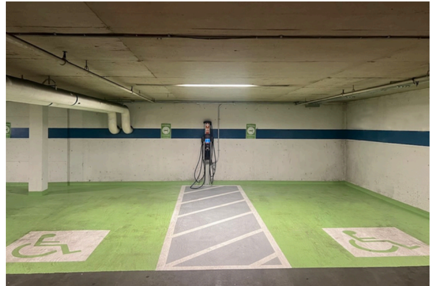
Figure 2 - SFU has opened our first two accessible EV charging stalls on campus.
