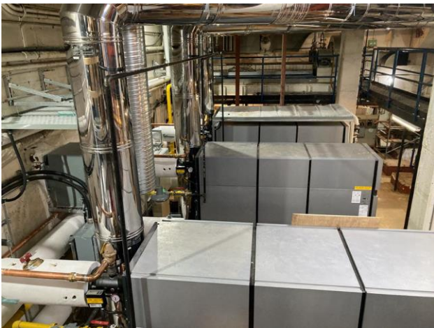
New gas boilers at St. Paul's Hospital
