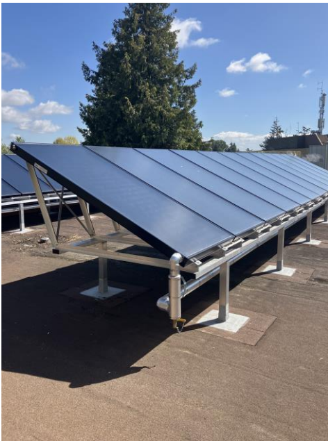
Photo 1: Delta Hospital Solar Thermal Panels
