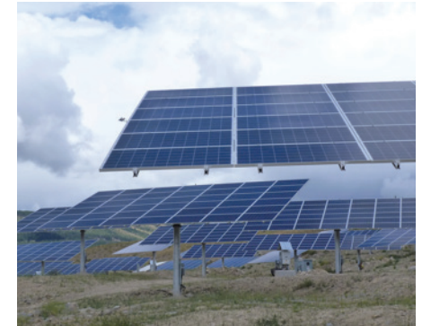
SunMine, in Kimberley B.C., provides 1 megawatt peak production, enough to power about 250 homes, and was the first solar project in B.C. to sell power to the BC Hydro grid.
