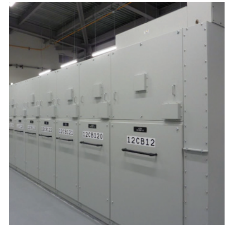
Capilano Substation Dry-air medium-voltage switchgear system
