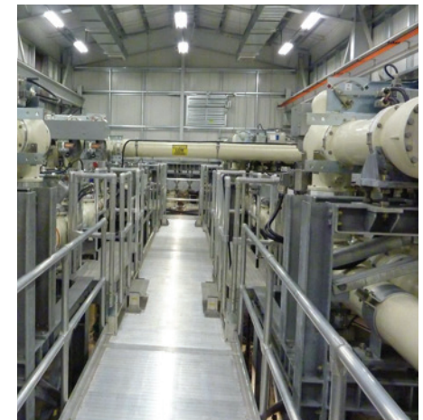
A 230 kV Gas Insulated Switchgear (GIS) unit in Horsey Substation
