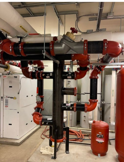
Photo 2: Re-piping work of the heat pumps and boiler circuits before insulation was applied.
