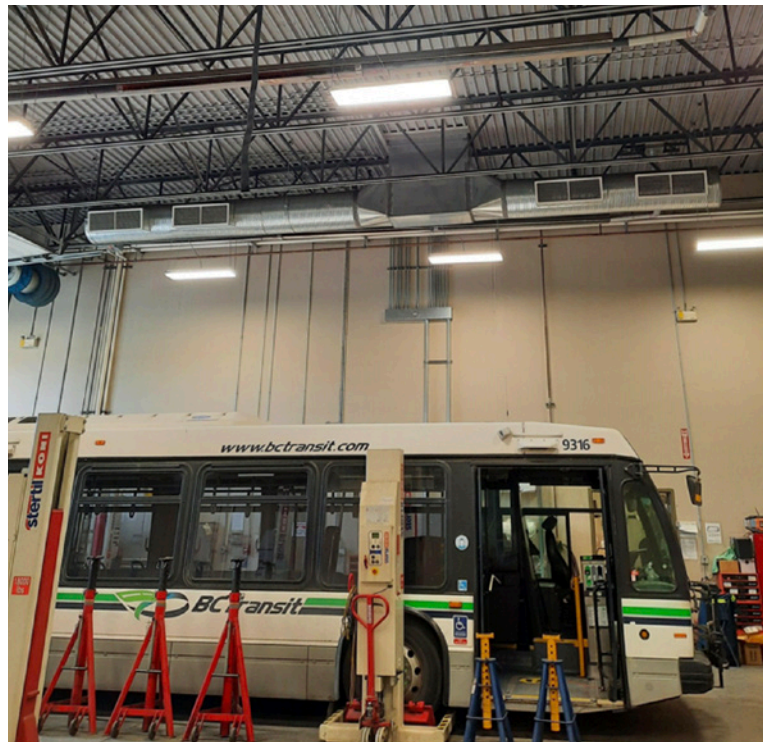
Chilliwack Transit Centre Bay Lighting
