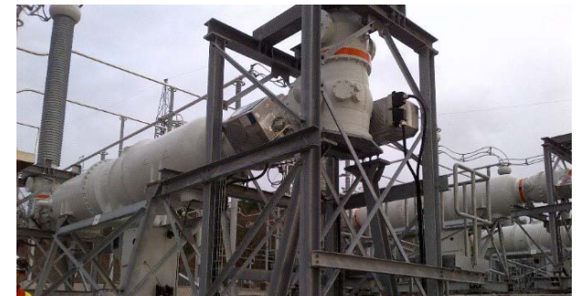
Medium Voltage Circuit Breaker
