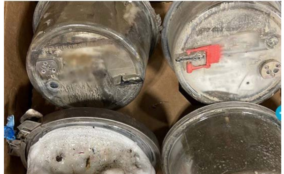
Electrical meters that were removed from flood-affected buildings following the atmospheric river weather event.
