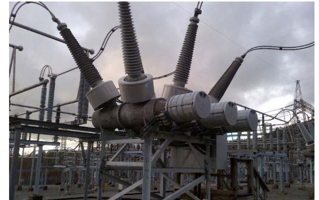
High Voltage Circuit Breaker
