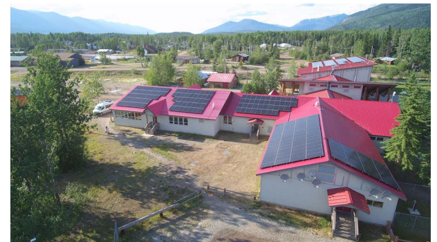
Kwadacha Aatse Davie School Solar System by Green Sun Rising Inc.
