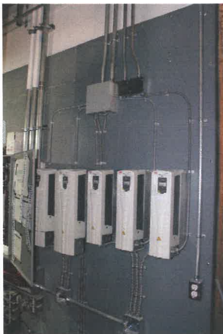
New Mechanical Systems—state of the art Variable Frequency Drives (VFD)
